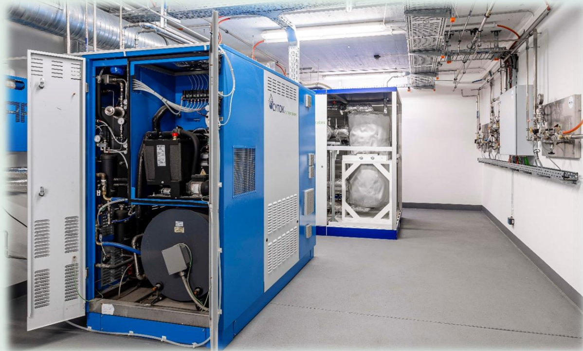
CYTOK Power-to-Gas Anlage
